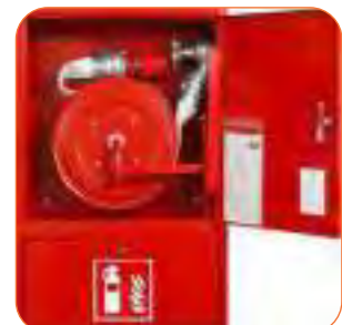
Fig 11.2.14 Fire hose cabinet
